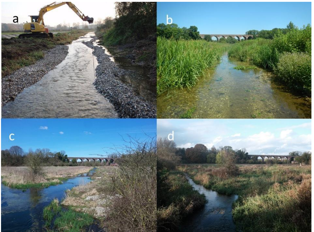
Figure 11 BREC facing downstream while undergoing channel reprofiling in 2009, the straight and wider profile of the channel can be seen beyond the mechanical digger, and the newly contoured profile in the foreground (Image: Simon Cain, reproduced with permission) (a), looking upstream reach from the furthest downstream point in June 2018 (b), looking upstream from below the confluence with BRWC (on the left) following annual weedcutting in April 2018 (c) and having become infilled with emergent macrophytes in November 2018 (d)
