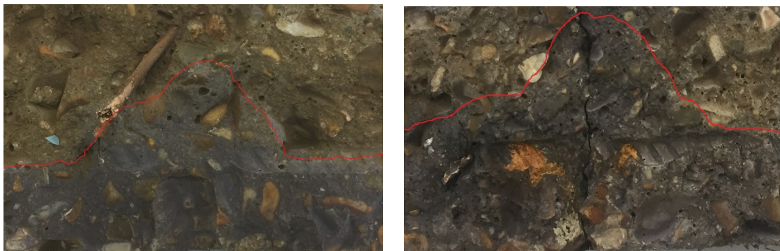
M 0.4-crack width 0.1 mm
