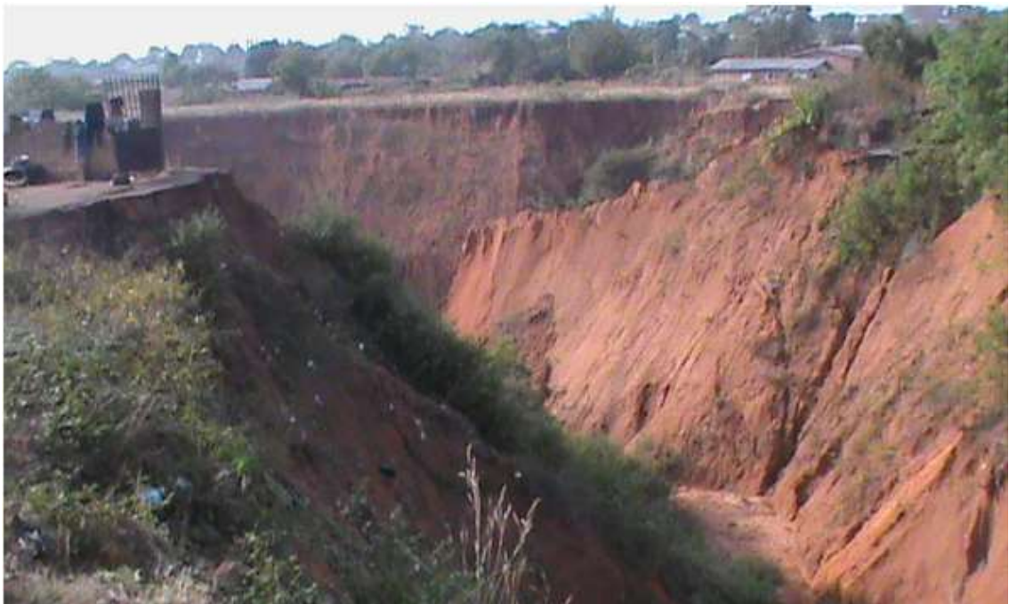
Figure 32: Active gully-walls of Njaba Gully site
