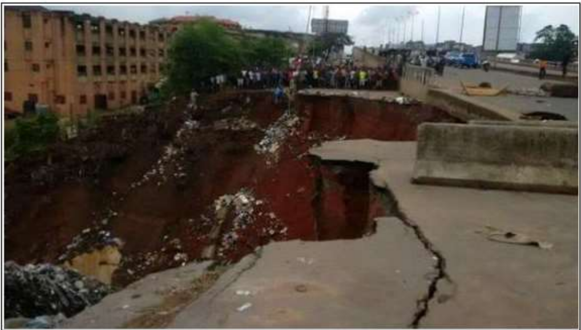
Figure 6: Nkpor gully site (Onitsha – Owerri Road) southeast Nigeria.
