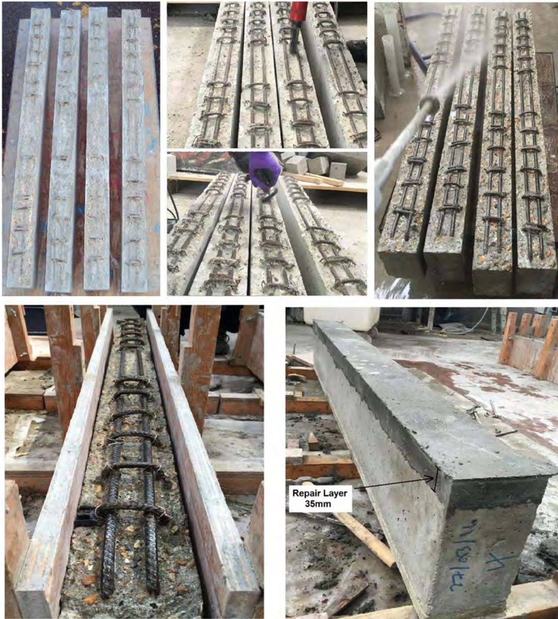
Figure 8.4 Preparation the surface of RC concrete substrate and casting the repair/strengthening layer.
