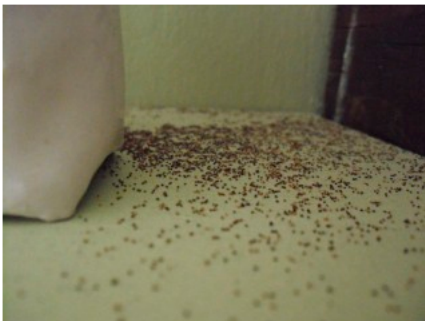
Figure 98: Borer dust on a shelf, Durban, South Africa. Photo: C. Bagley 2011.
