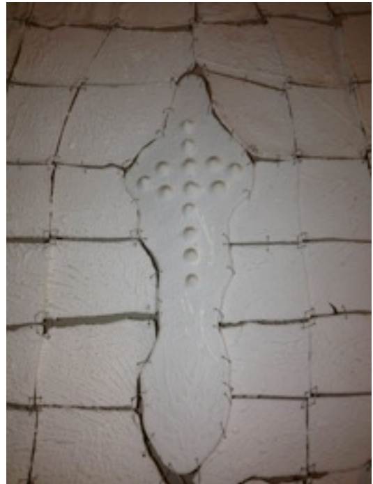
Figure 38: Detail of Figure 37. Photo: L. Frisinger, 2012.
