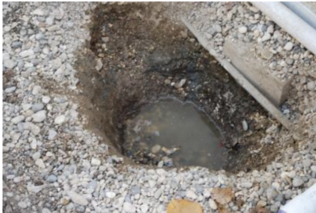
Figure 2.5: High groundwater level at the MSF hospital site in Port-au-Prince: the traditional approach for wastewater disposal was therefore not applicable
