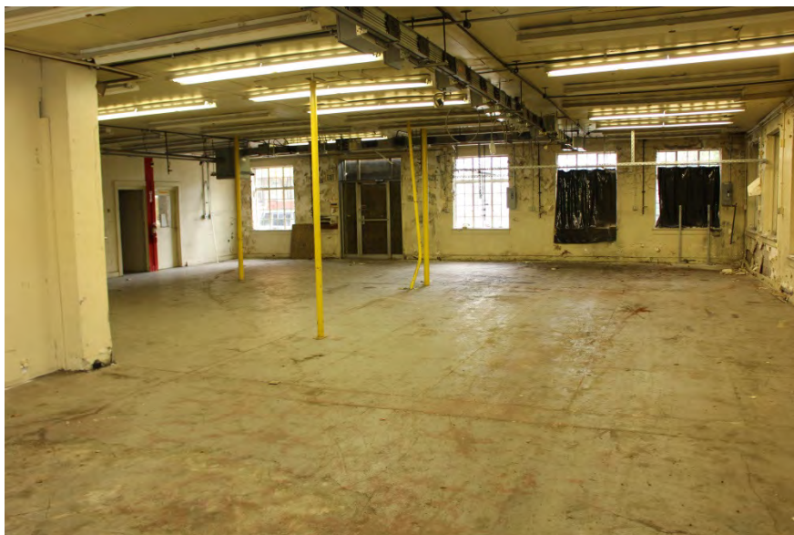
Figure 74: Interior aspect of entrance area of one of The Tube warehouses (pre-renovation), Indianapolis, 2014. [Photograph].
