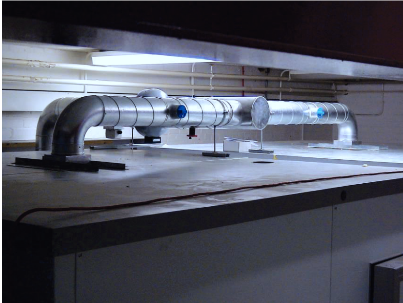
Figure 8.3 Photograph of air-conditioning installation to the environmental chambers
