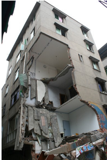
Fig. (16). A partial collapsed 6-storey building due to collapse of load-bearing masonry walls at Mianyang city.
