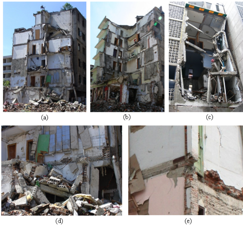
Fig. (12). Damage of confined masonry buildings (a), (b), and (c) partial collapses, (d) collapse of simply supported hollow precast slabs, and (e) pullout failure of a beam.
