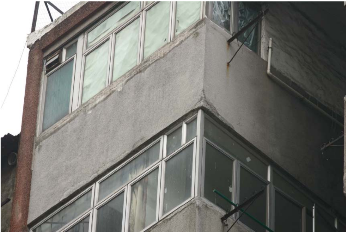
Figure 2.13 Photo showing water leakage problems at window in an old building
