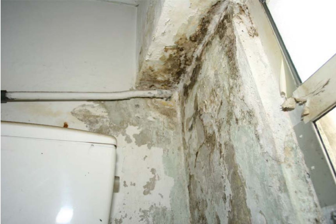
Figure 2.12 Photo showing water leakage problems inside an old building
