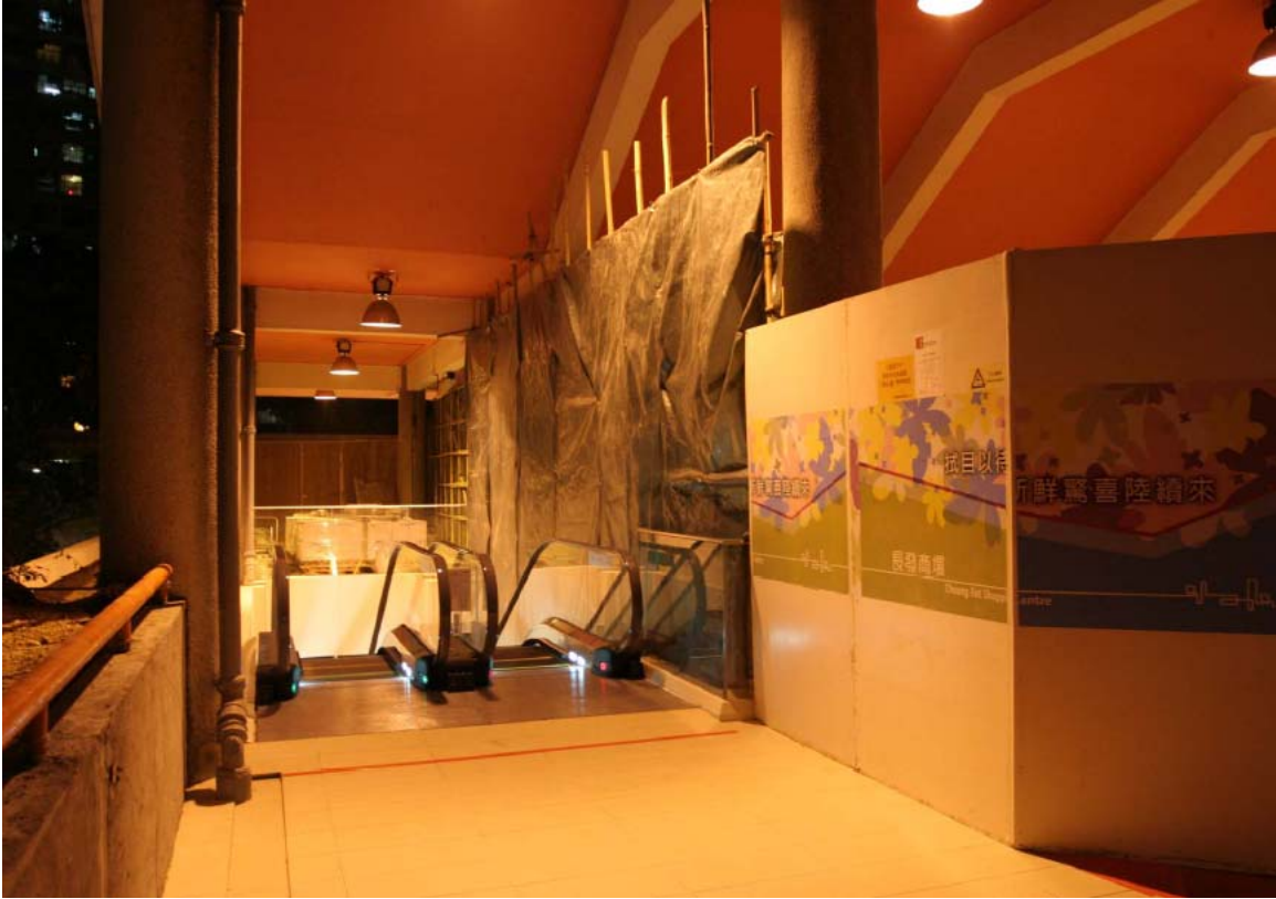
Figure 4.4 Application of machineries to enhance maintainability depends on specific cases: mechanized platform cannot be used over escalator
