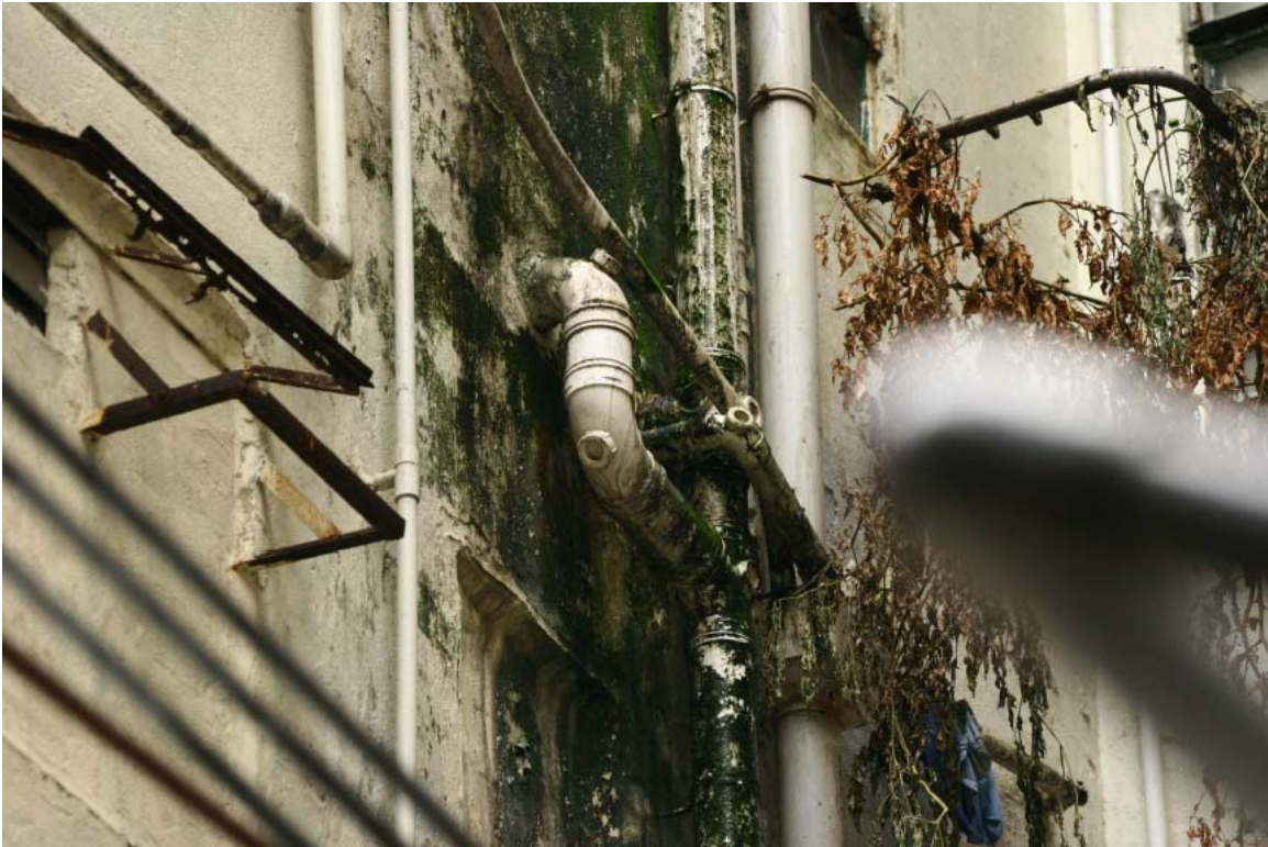
Figure 2.19 Fungi and algae growth around leaked pipes
