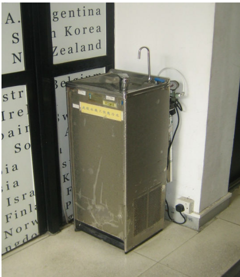
Pic. 71: Water Fountain at SWH
