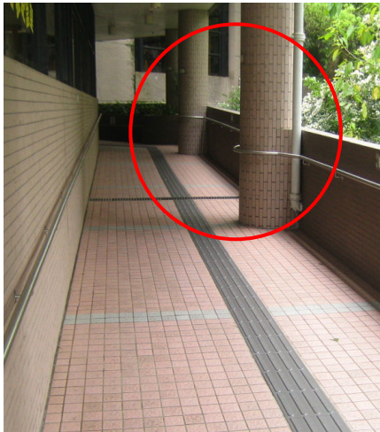
Pic. 65: Protruding Elements along Ramp to KK
