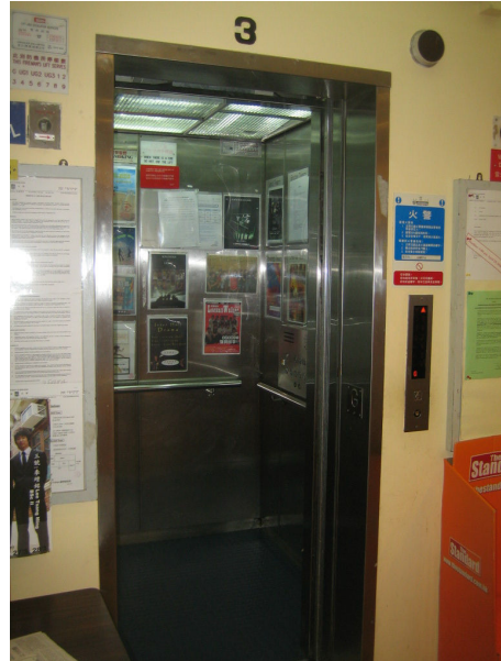
Pic. 2: Lift Serving Every Floor of COB on G/F of Simon K.Y. Lee Hall
