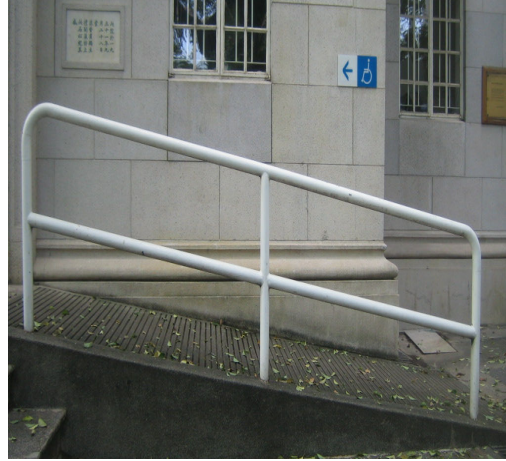
Pic. 74: Too Steep Ramp at Entrance of TC
