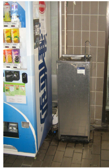
Pic. 68: Water Fountain
