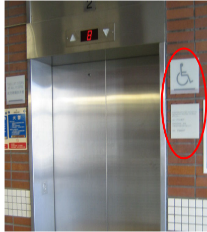
Pic. 36: Lift Designated for Wheelchair-bound Persons
