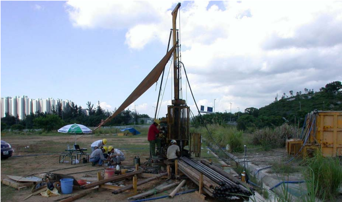
Figure 1. Hydraulic rotary drilling machine equipped with drilling process monitor for ground investigation
