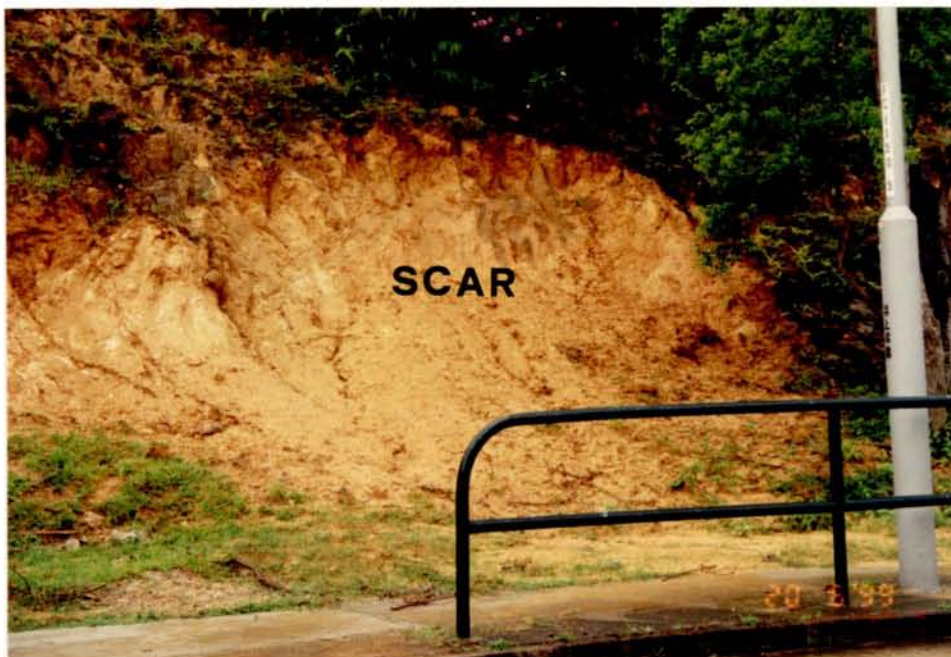
Plate 9.4. Landslide along a roadcut at South Lantau Road exposing deeply-weathered reddish-brown soil.
