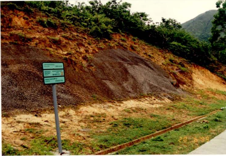
Plate 9.7. The roadcut slope was not properly protected by shotcrete, at South Lantau Road
