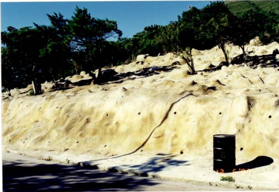
Plate 9.8. A newly-repaired roadcut slope with numerous surface drainage, at Tung Chung Road
