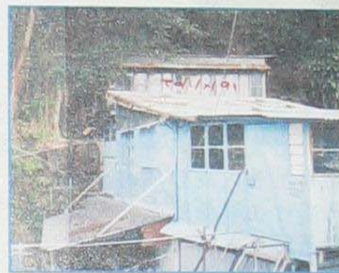
脆弱的寮屋結構 Flimsy squatter structure
