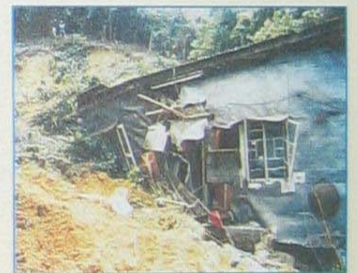
受山泥傾瀉毀壞的寮屋 Squatter hut damaged by landslide
