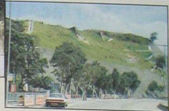
坡腳種植大樹遮擋噴漿混凝土護面 Large trees at slope toe to screen the shotcreted surface
