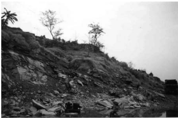
Fig. 7. A side view of the landslide debris comprising mainly weathered mudstone, looking south. Thick sandstone can be seen underlying the deformed weathered mudstone, and seepage from the contact bedding interface between the weathered mudstone and the sandstone is also visible.
