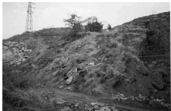
Fig. 5. The landslide debris comprising mainly weathered mudstone that travelled about 13 m onto the platform for the road subgrade, looking NE. Thick sandstone can be seen in an adjacent cut slope below the transmission tower.
