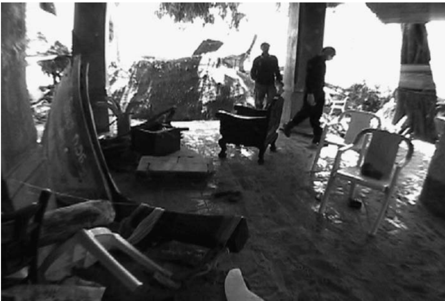
Plate 5. The wooden posts of the banyan tree lobby in Phi Phi survived even after being hit by a boat because the ground floor was open, allowing wide and shallow flood flow
