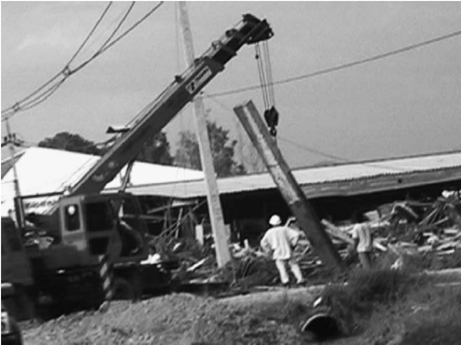
Plate 12. A power outage led to chaos and lawlessness. Debris tore down power lines
