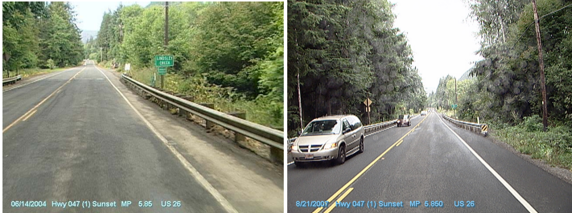
Figure 5.48: Conditions in 2004 (before) and in 2007 (after) showing the upgraded guardrail at Lindsley Creek BR 03095, MP 5.85
