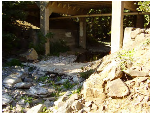
Figure 4.13: Site 10 – Chenoweth Creek failed under-structure concrete lining
