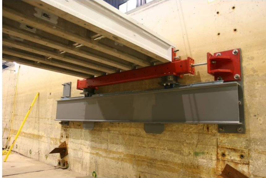
Figure 3.6. Photo of rigid test setup installed in Large Wave Flume. In this photo, the horizontal load cell between the bent cap and the end anchorage block has been temporarily replaced by a 1-inch threaded steel rod.
