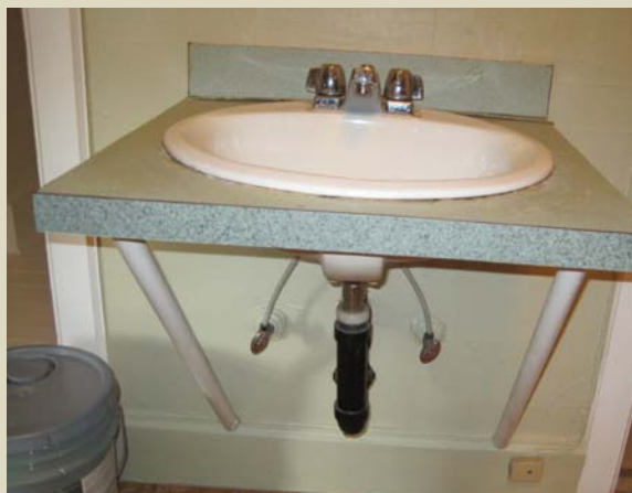
Sinks in units
