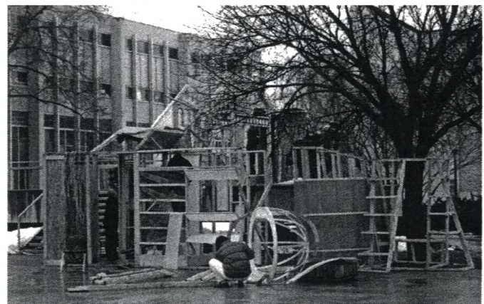
Fig. 2. The individual 4' x 4' x 8' cells being assembled as part of the entire structure.
