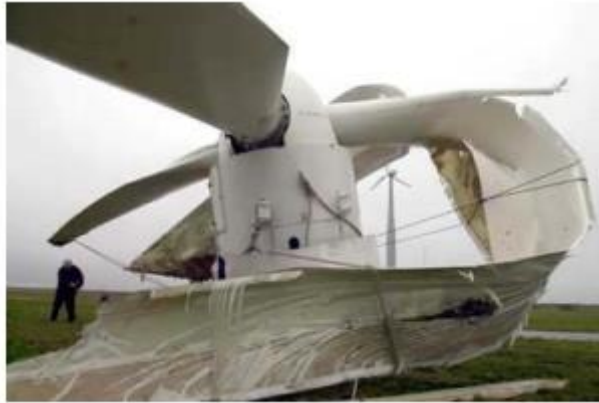
Figure 11: Catastrophic failure of wind turbine blade due to manufacturing induced defects. Taken from [94].
