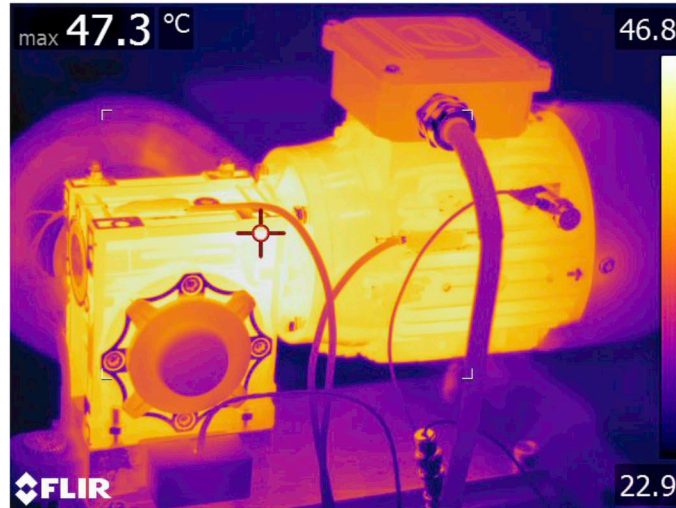
Figure 7.10: Thermal image of CER drive system during unloaded operation at 45Hz.
