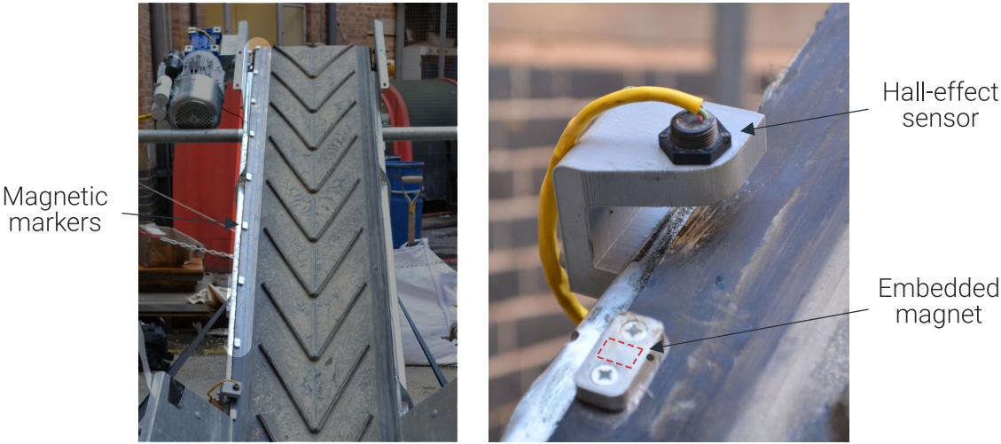
Figure 8.6: Bespoke belt speed monitoring hardware.
