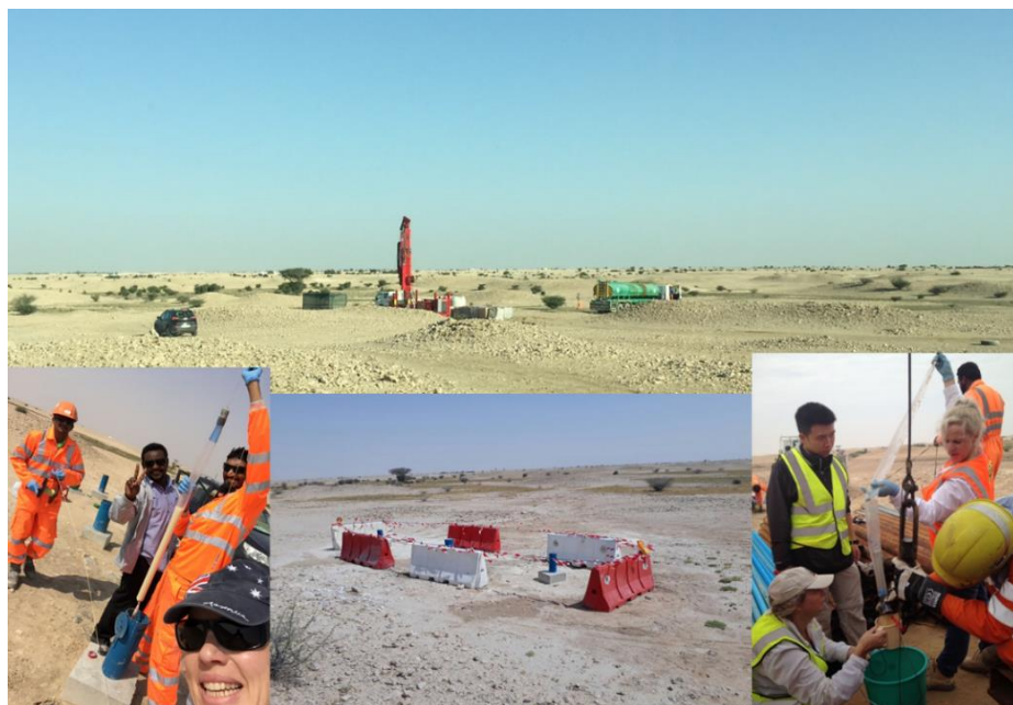
Figure 3-1 Drilling of RR (southern) wells and surrounds, monitoring, and wells on completion
