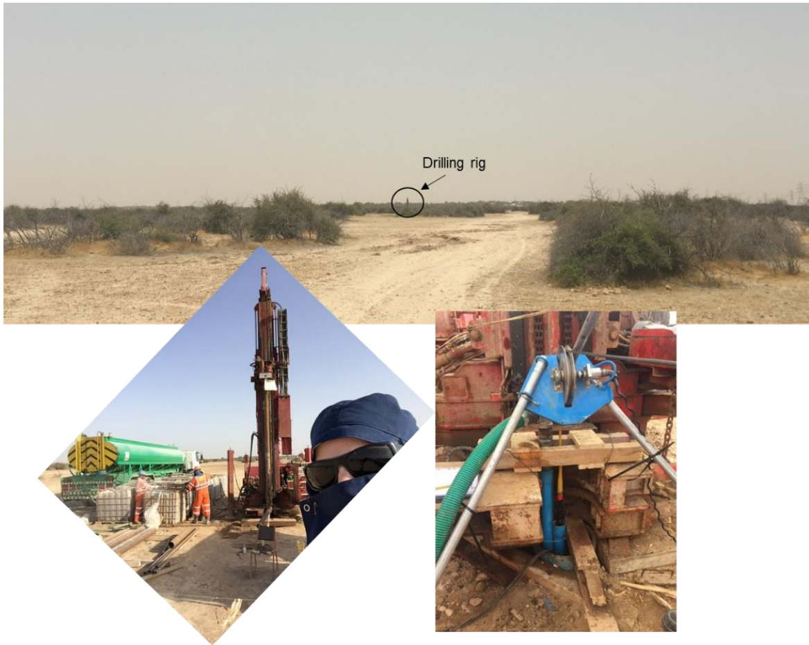
Figure 3-6 Northern (AG) well surrounds, site crew during drilling and geophysics down-the-hole temperature and EC probe attached to tripod winch
