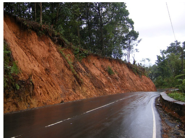
Fig. 1 Road cut slope, Saint Lucia primary road network, after landslide debris cleared (photo: E A Holcombe)
