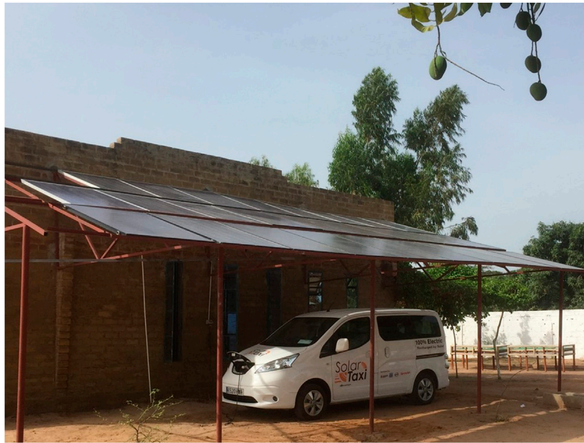
FIGURE 4 | The Solar Taxi recharging from the minigrd at Manduar that is powered by a 4.5 kW PV array that forms part of the roof of its car port (Source: Gammon, 2019).
