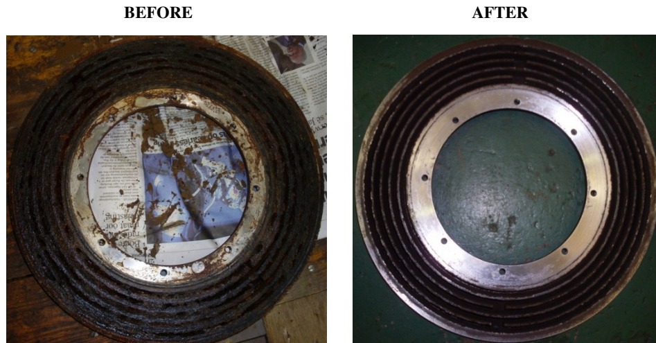
Figure 49: Loss plates before and after cleaning
