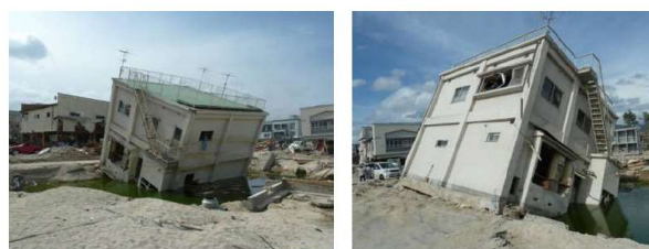
Figure 3 - The failure mode of building foundations shows tilting leading to rotation and collapsing due to a large scour hole
