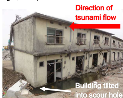
Figure 1 - Apartment block scouring at the seaward end in Yuriage, Japan due to the 2011 Tohoku tsunami (Fraser et al., 2013)
