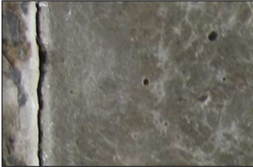
Figure A14: Debonding of concrete form mould side
