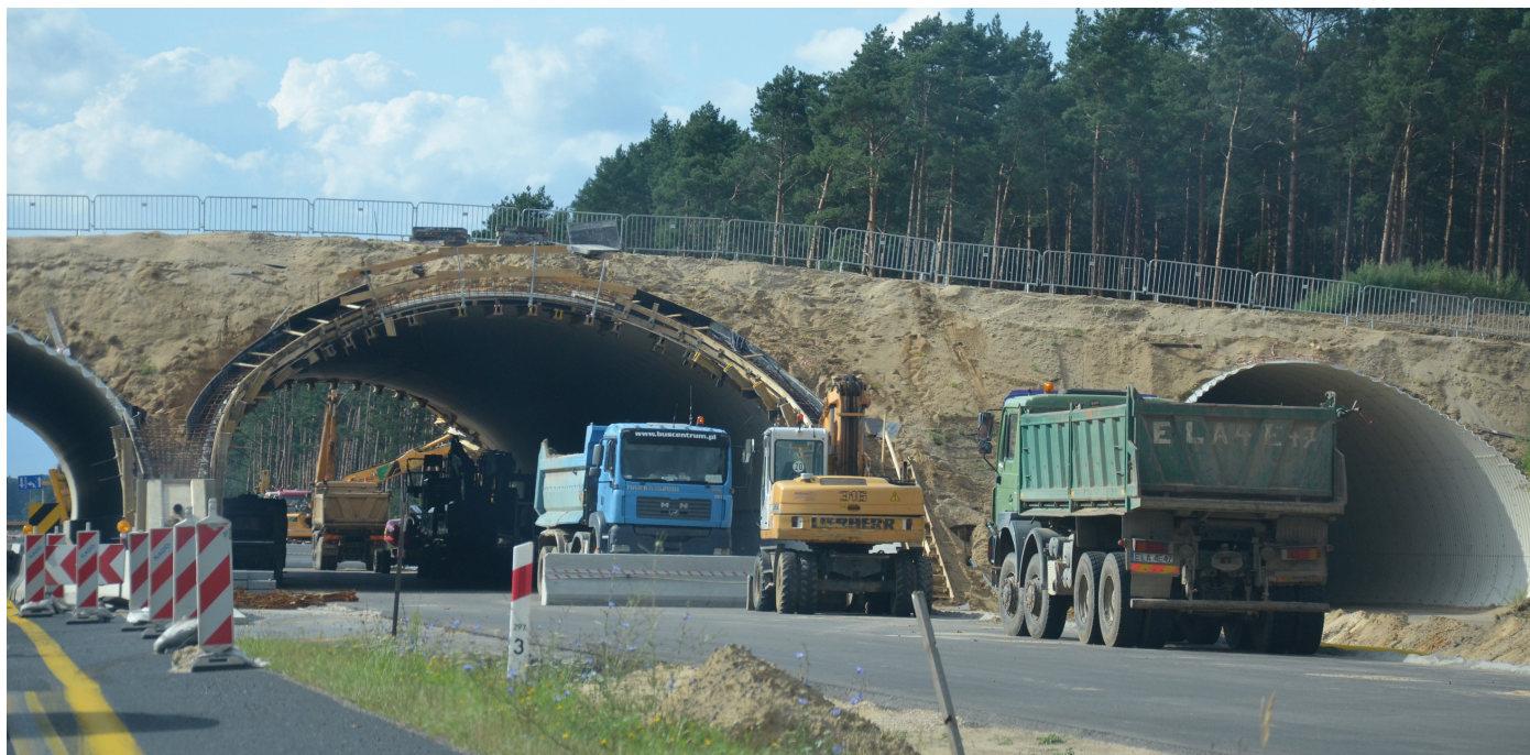
Fig. 3. Thick heap material in the road flyovers – stored directly on earth surface (embankment) or isolated from the surface, i.e. over the constructed tunnel (photo A. Greinert)
