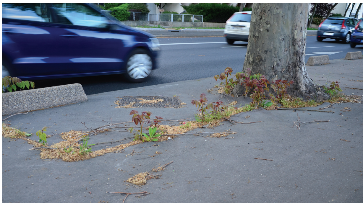
Fig. 5. Cracked, discontinuous surface of Ekranosol destroyed by plant roots (photo C. Kabała)
