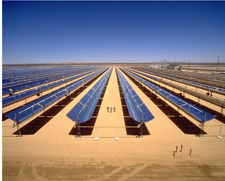
Figure 2.6: SEGS III parabolic trough plant at Kramer Junction, California [62].
