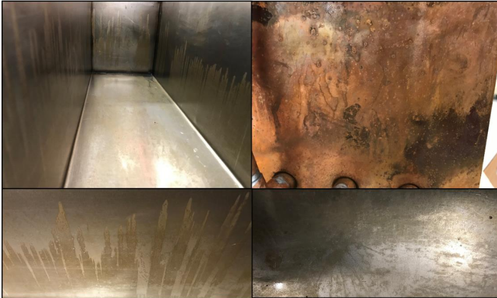
Figure 5-20: Pitting on the surface of the mild steel container and copper fins
