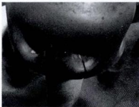
(c) Cover damage
