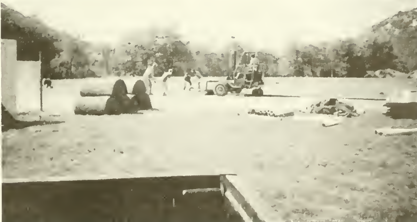
Ongoing work at Memorial Field, part of the Eli Isaacson Sports Complex
