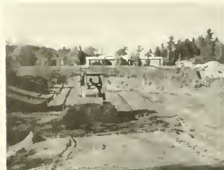
Fall, 1987 construction of shallow lagoons for chemical waste water storage at East Milan Road Water Treatment Facility.
