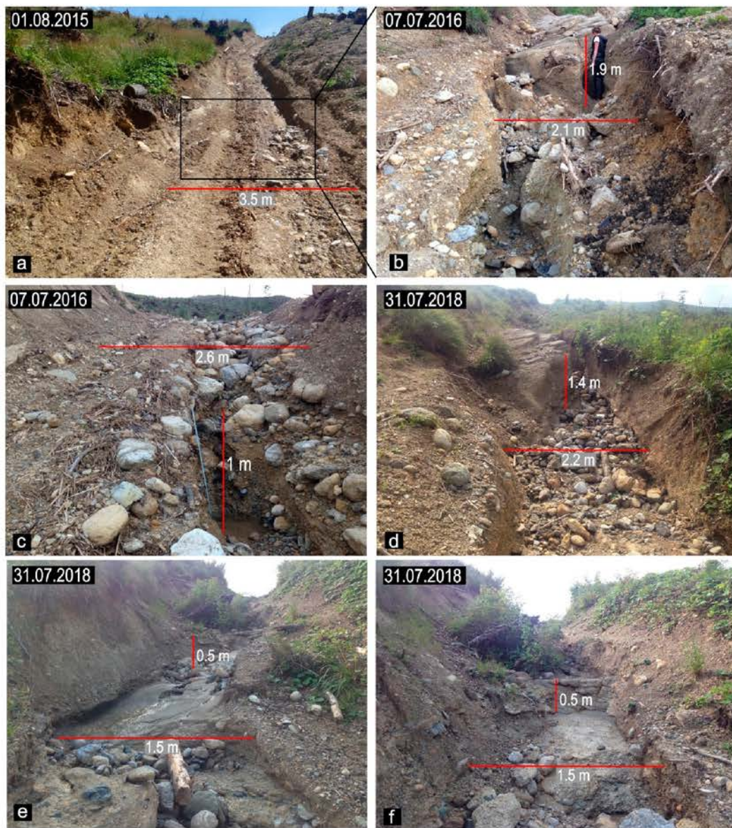
Figure 2. Changes on the surface of the studied road, explanations: the road in use in the first year after its construction (a); deep incisions formed after heavy rainfall, which contributed to exclusion the road from usage (b,c); strong relief transformations on the road two years after exclusion the road from usage (d–f).
