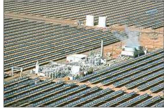
Figure 12: Parabolic trough plant, Boron, California 31
