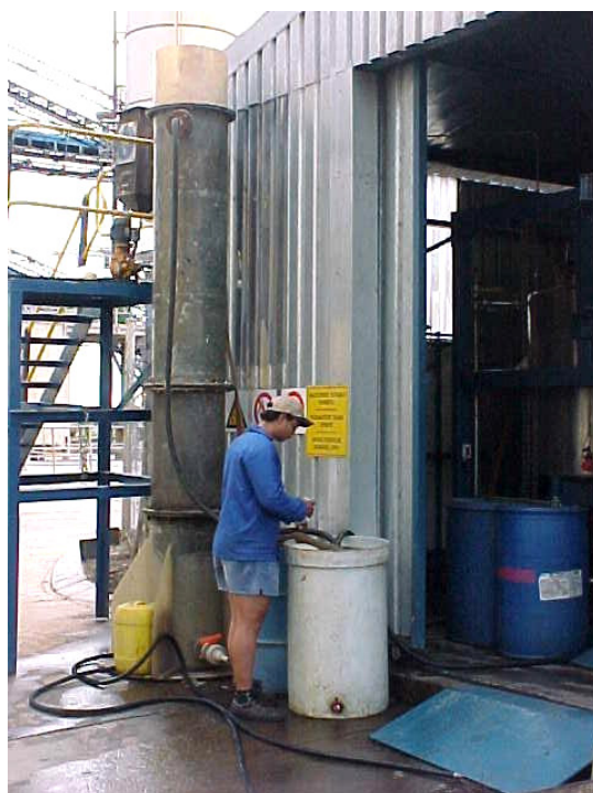
Figure 5.15: The E-CAT™ clarifier installed at the pilot plant
