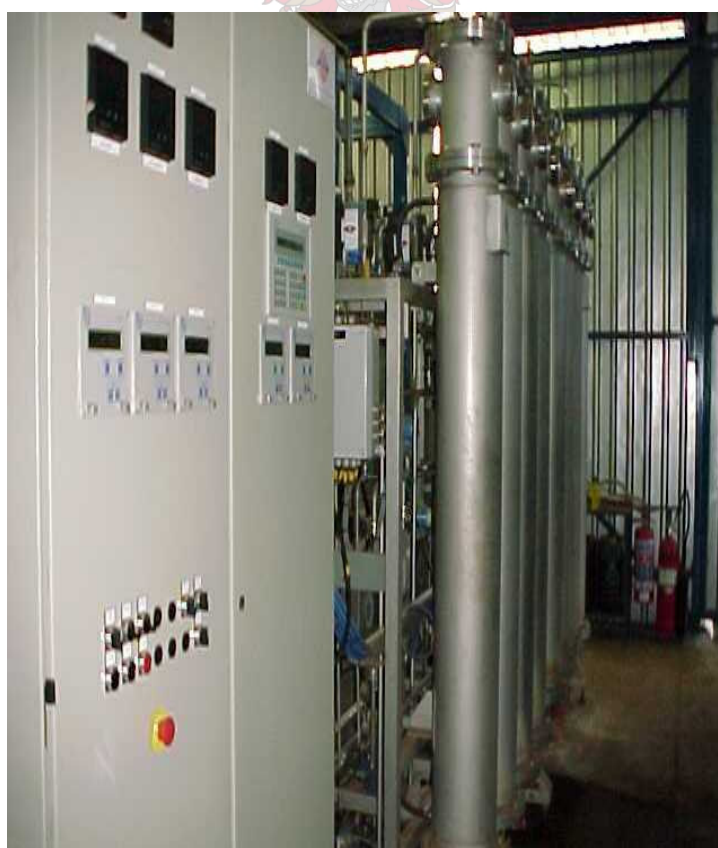
Figure 8.2: The Chromatography Pilot Plant. The control panel is visible in front and between the columns some of the manifold piping is visible.
