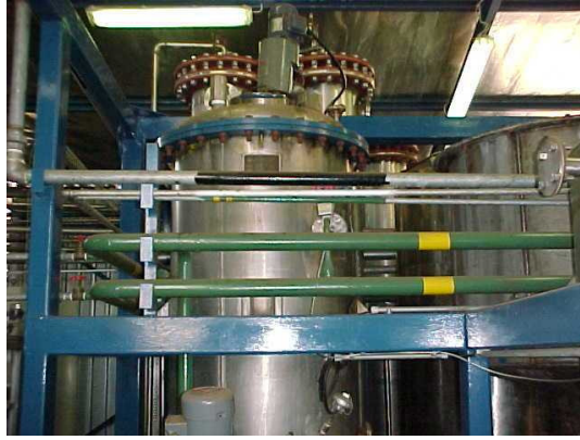
Figure 4.9: The chromatography feed tank with utility piping visible in the front. The deashing columns are at the back.
