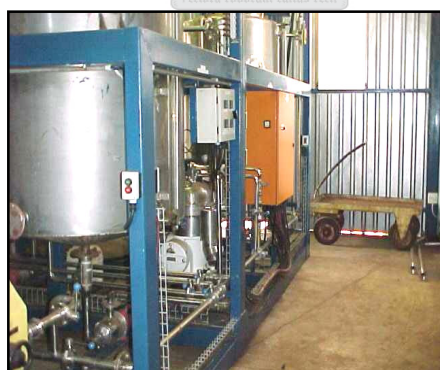
Figure 5.3: A view of part of the molasses pre-treatment pilot plant. The tank at the back is the dilution and centrifuge feed tank. The centrifuge is the white and shiny object in the centre. The tank in the foreground is the filter feed tank. The orange enclosure houses the electrical panel.
