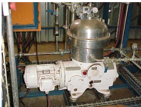
Figure 5.2: The Westfalia Disk Bowl Separator seen from the operator side. The feed and product pipework is visible at the back and the water pipe used to open and close the bowl is visible in the front. Sludge discharge is behind the unit on the right hand side.
