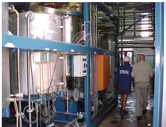
Figure 4.11: Skid 2 with the inversion reactors in front and the utility supply piping can be seen above the personnel.
