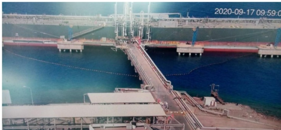
Figure 7: Floating boom on the oil terminal
