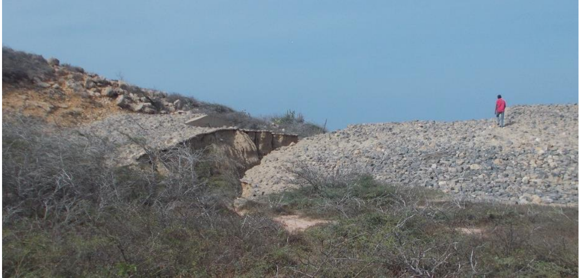
Figure 15. The collapsed Putaimaru Dam in 2017
