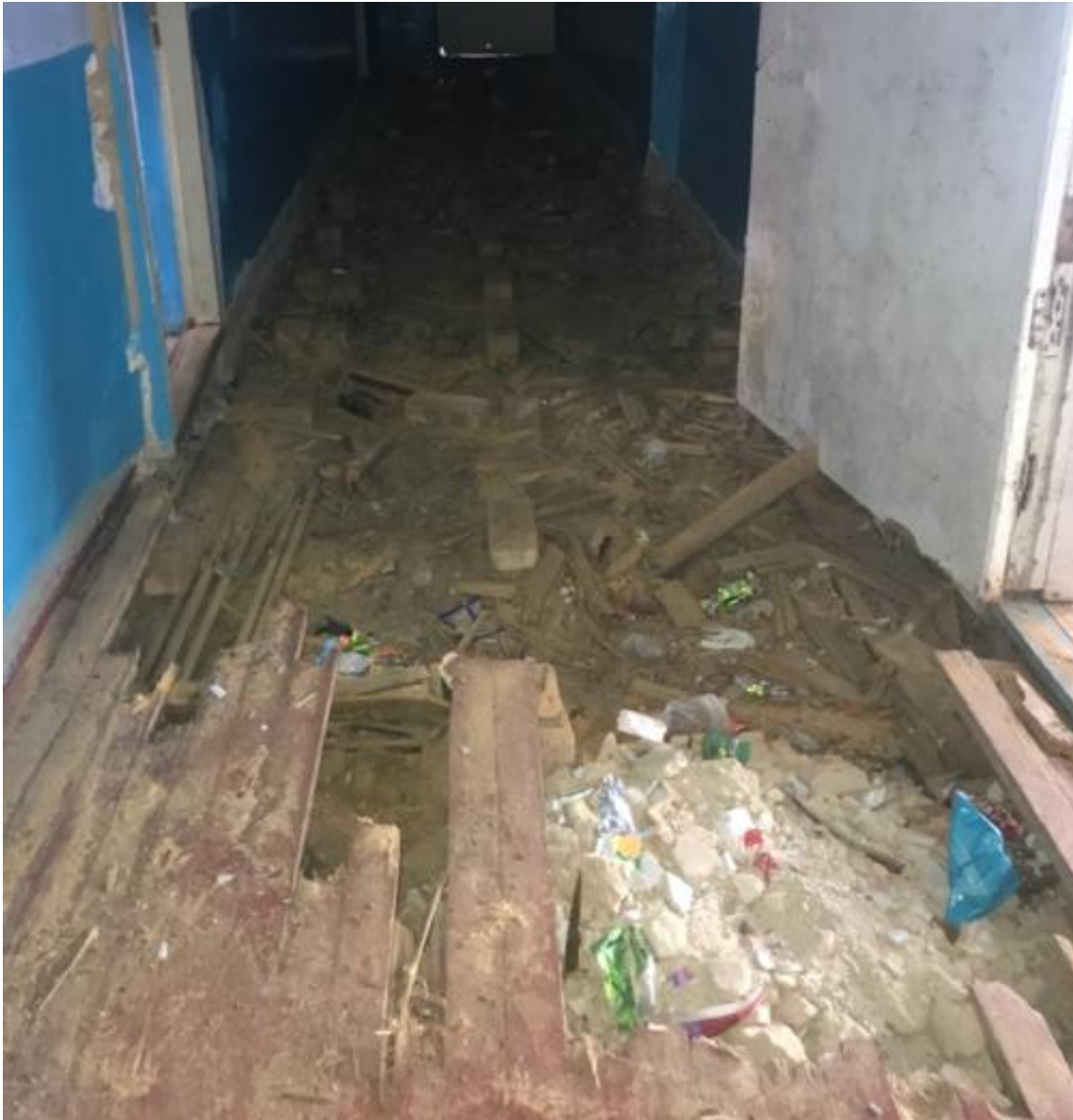
Figure 3: The image shows the condition of the access hallway to the gym. As shown in the image, the floor is rotten and in most areas missing.
