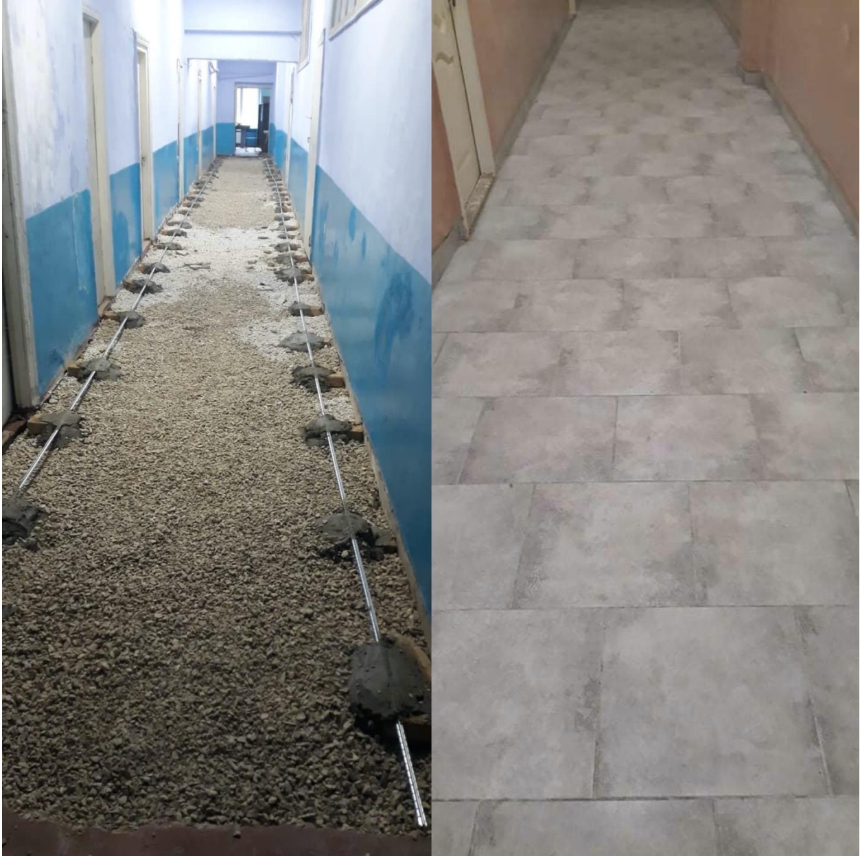
Figure 5: The image shows the access hallways after the rotten floors were removed. The floor was leveled and filled in with gravel and then concrete was poured over. Durable tiles were added along with a new coat of paint.
