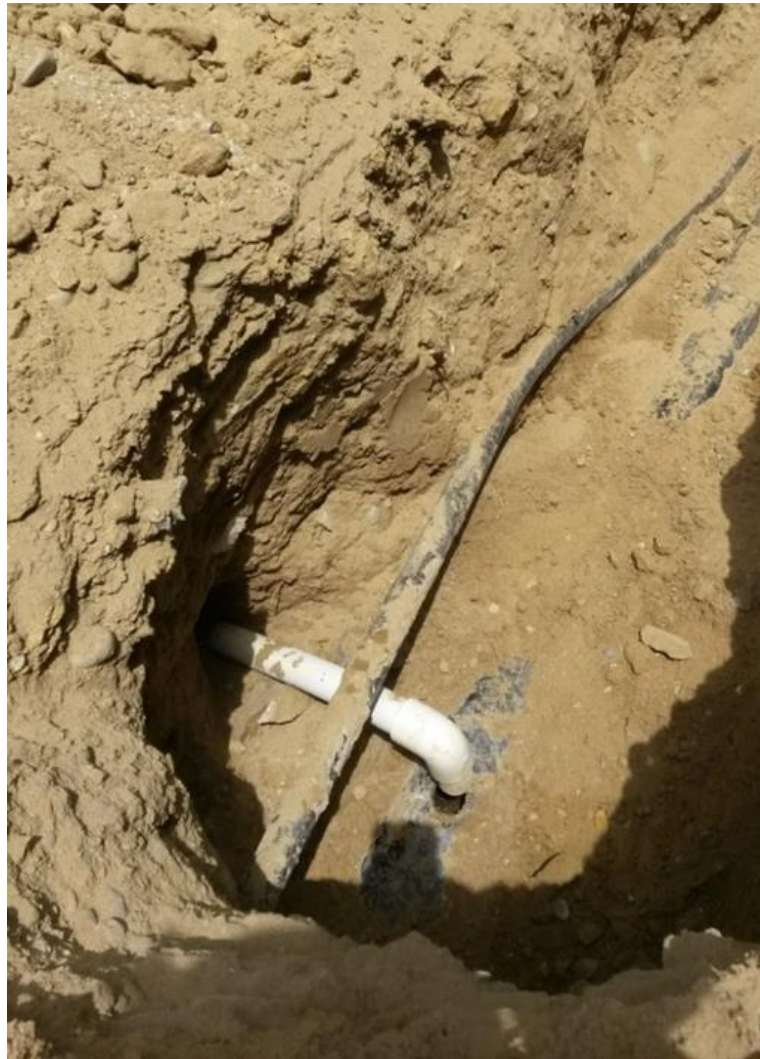
Figure 4. 1: Elbow joint connecting houses to the supply system (photo by author)
