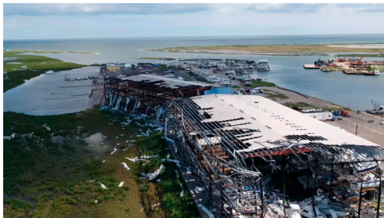
Figure 1. Unpiloted aerial system (UAS) data acquisition after Hurricane Harvey in Rockport, TX, USA.
