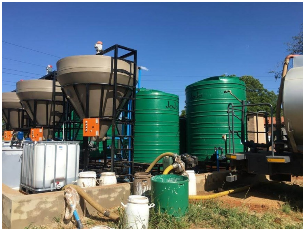
Figure 7: The treatment plant at within CSIR premises in South Africa
