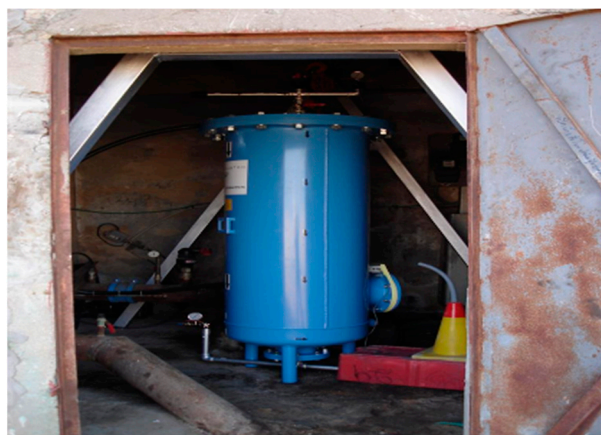
Figure 6. Pilot in a Yashresh well.
