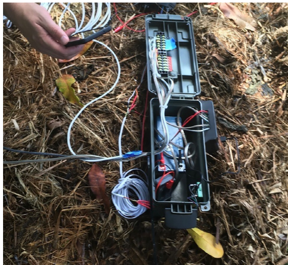
Fig. 1. Assembled ammo-can battery box deployed in Hilo, Hawai'i. Shown with lid open.
