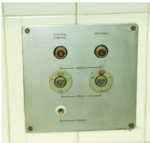
Figure 7-8: Control panel for the CCTV network in the anatomy dissection laboratory ©VHMD
