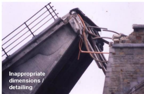
Bridge collapse (Melle 1991)
