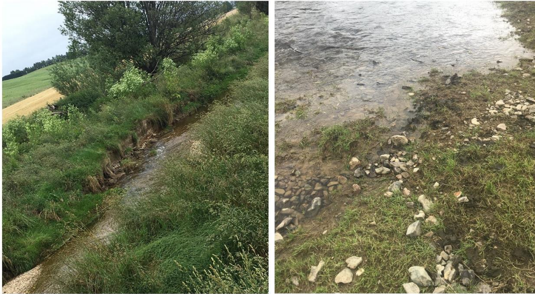
Figure 5.3: Photograph of Site 9 (left) showing a bank collapse on the true right side of the stream, and Site 3 (right) showing direct animal faeces in the waterway because of unfenced stock near the stream.
