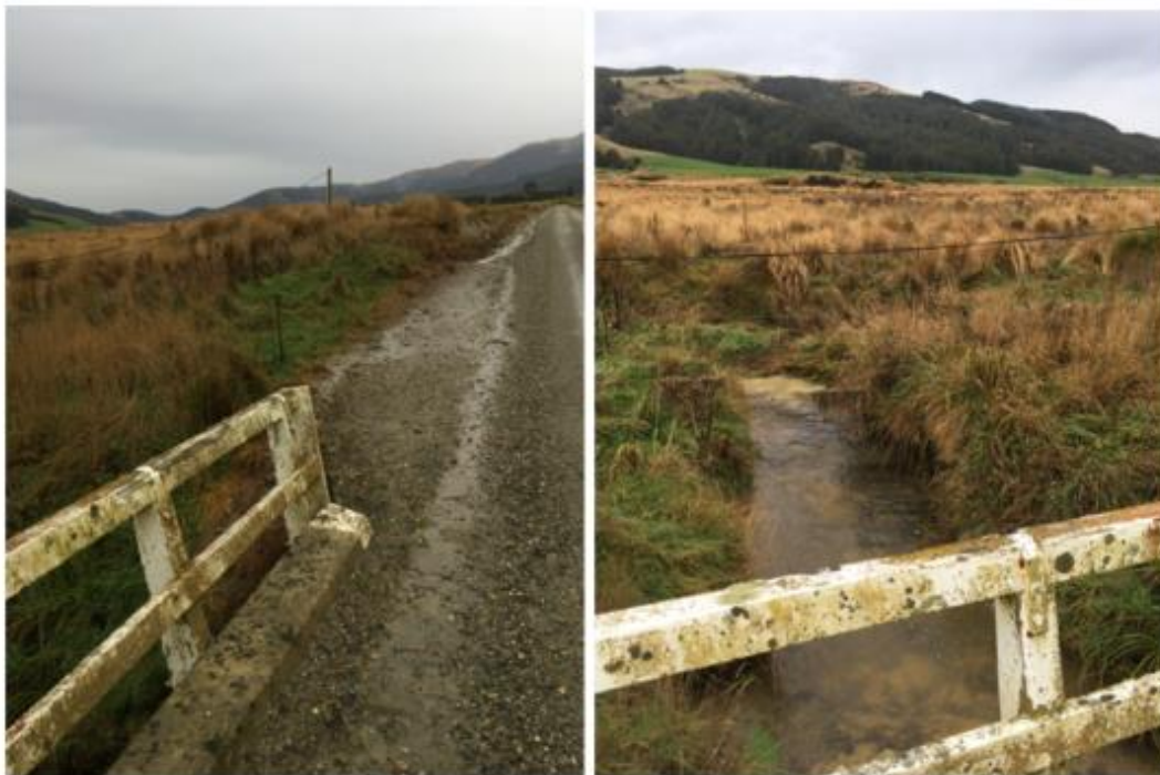
Figure 5.2: Photographs show an unsealed road at the top of the Waikaka Catchment during rainfall. The sediment can be seen running off the side of the road, and directly entering the stream, causing a plume of dirt in the water.
