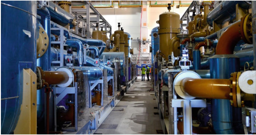
Fig. 26.16 Cryogenic system installed in buildings 51/52
