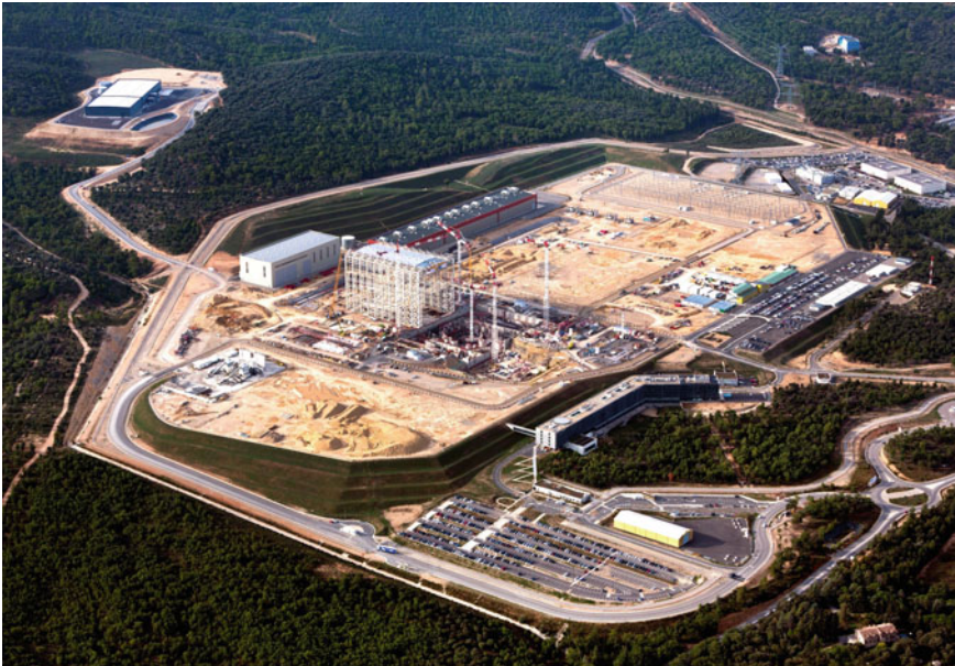
Fig. 26.2 Aerial view of the ITER site at St-Paul-lez-Durance with the construction of the Assembly Hall and Tokamak Complex
